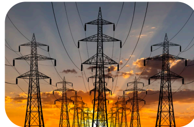
Utilities Micro Grids Renewables
